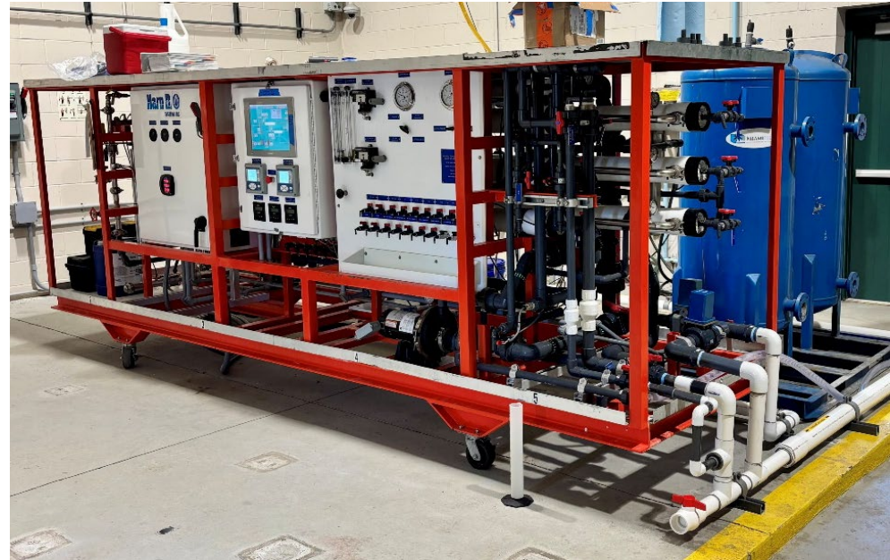
Reverse Osmosis Skid System
