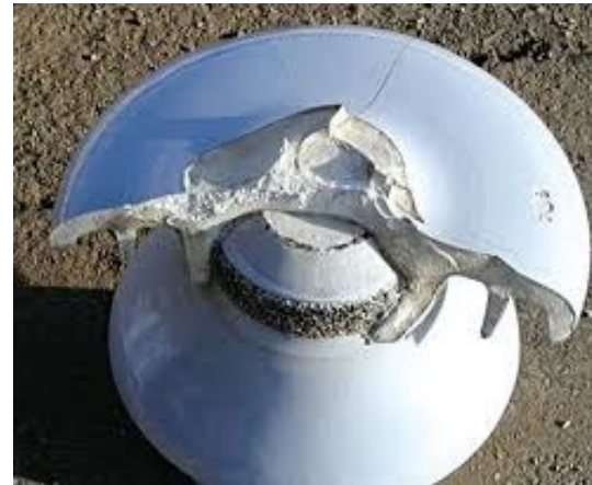
Broken 12kV porcelain insulator
